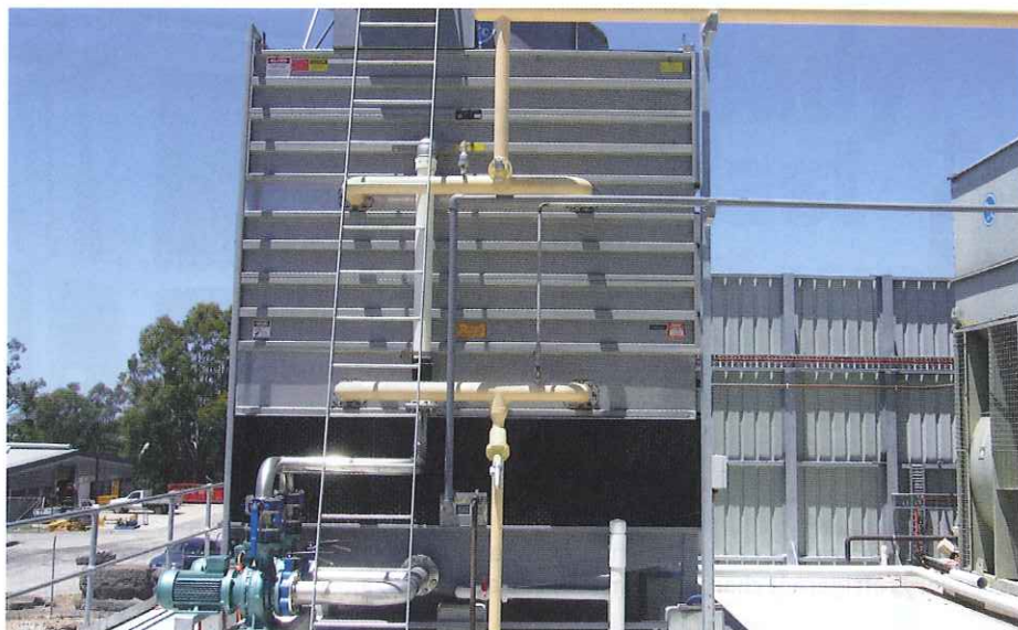
An evaporative condenser with variable speed drives for fan and floating condensing pressure control.
