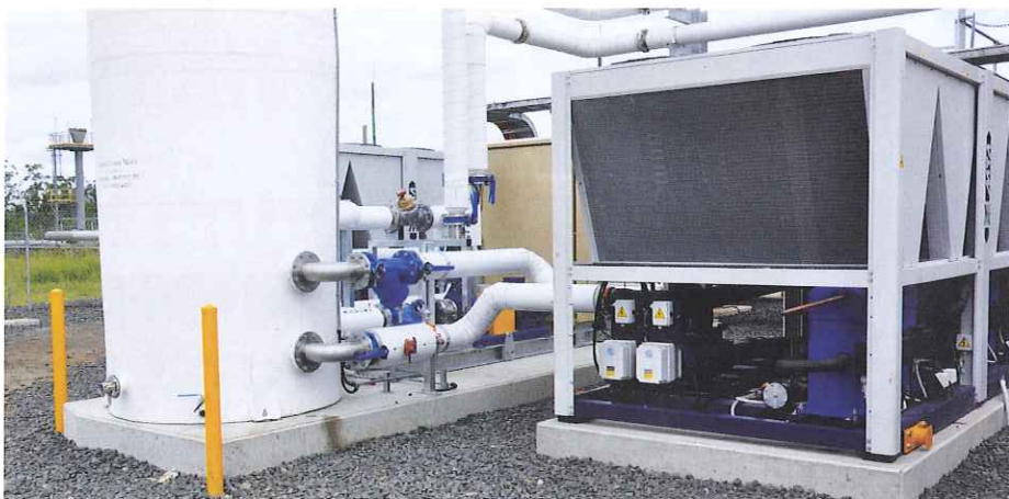
A packaged air-cooled chiller with multi-stage capacity control and large volume secondary refrigerant charge for smooth and accurate control.
